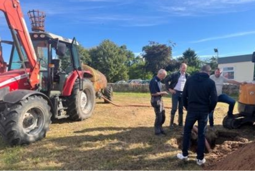
Excavation and percolation testing at one of several locations to determine drainage parameters
